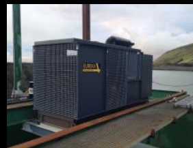
Hydraulic Power Pack
