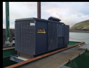
Hydraulic Power Pack
